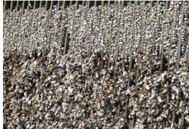
The zebra mussel can cause damage by blocking pipes, vents and any holes or openings where water flows. Reservoir tower safety grating clogged with zebra mussels (Rabisha Reservoir, Bulgaria).
