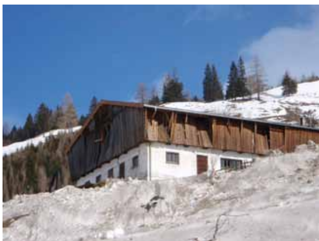
Figure 8.4 Building damaged by the Marchkar avalanche
