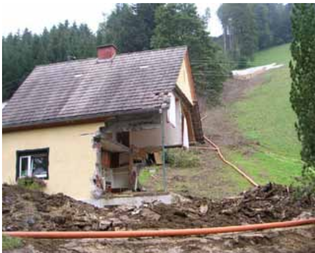
Destroyed house in which two people were killed Source: Andrecs et al., 2007.
