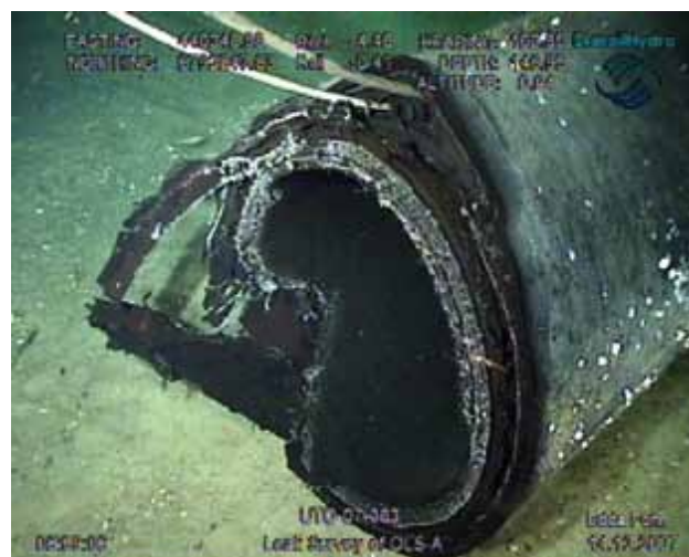
Figure 11.4 Picture of the ruptured loading hose
